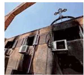
A view of the damage at the Coptic church in Giza on Sunday. • AFP
