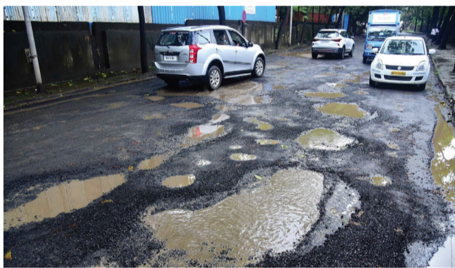
Plethora of potholes
